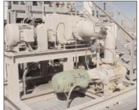
Booster blowers for deep vacuum.
